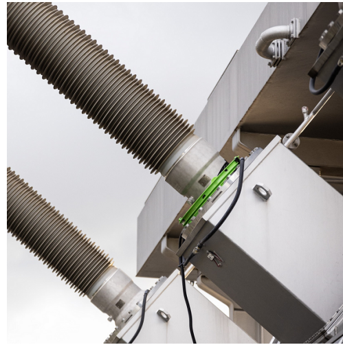
Figure 3. Installation of FOCS sensing head on one phase of a 380/220 kV power transformer in Vienna, Austria.
